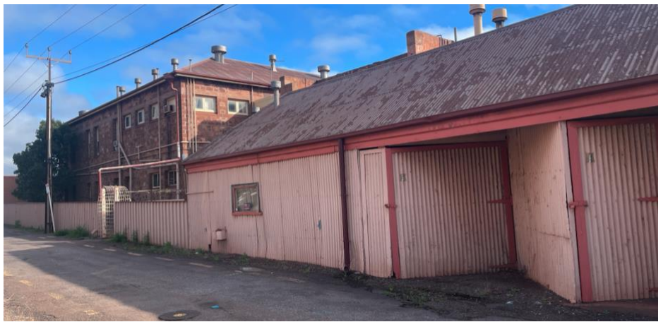
Figure 4: Spencer Hotel Balnaves (rear) Lane frontages showing structures proposed for demolition. DASH Architects, 2022
