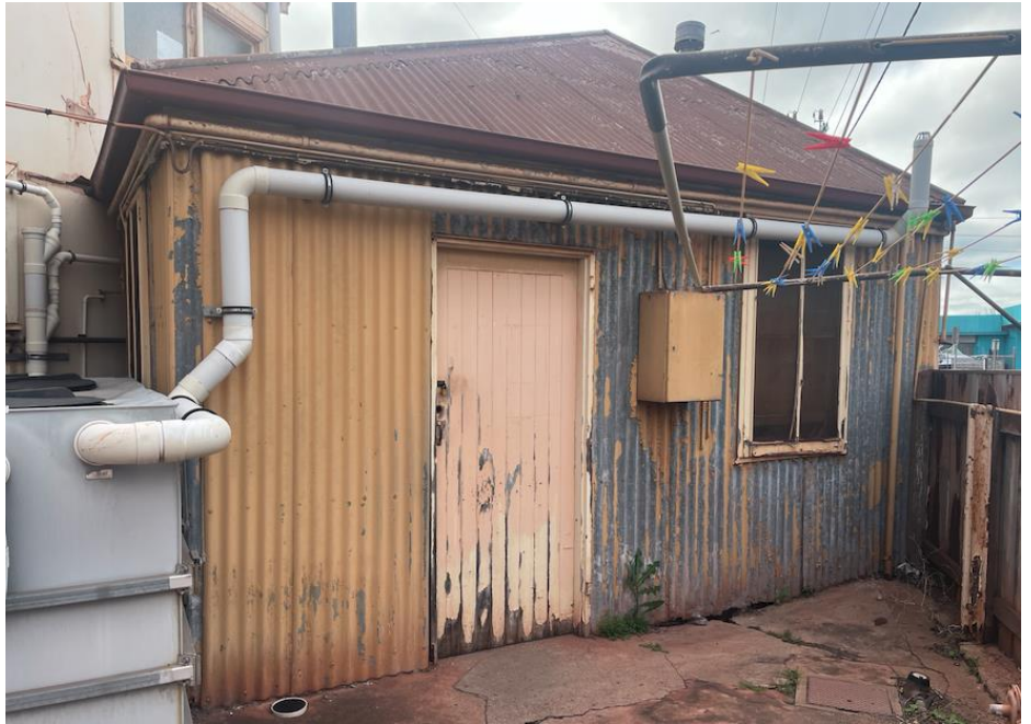
Figure 27: Former rear garage as viewed within site (identified with arrow). DASH Architects 2022
