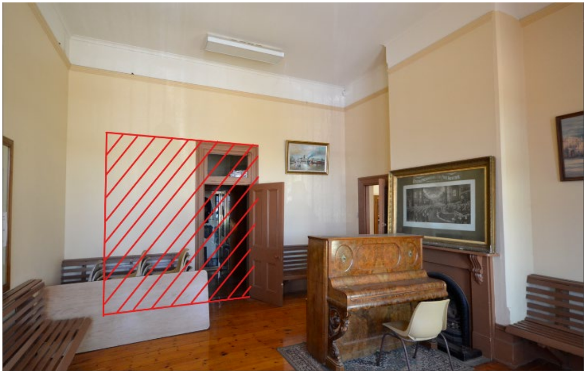
Figure 8: Indication of the extent of the proposed new opening to be formed between proposed Café space and Servery, maintaining existing opening height
