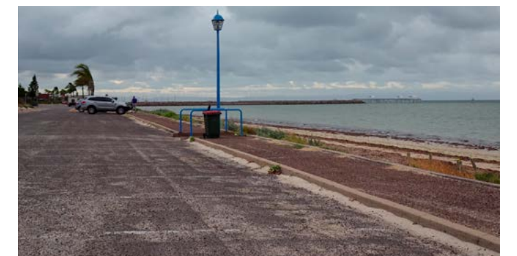
Poorly sealed car park at Western end of foreshore looking towards Jetty.
